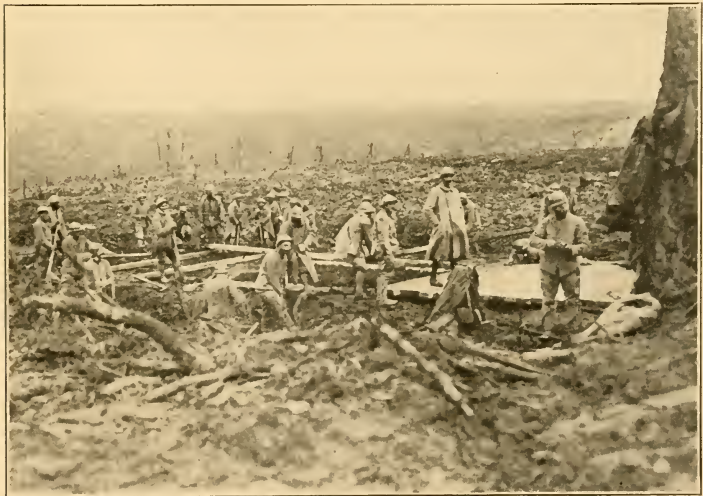
Near Moulin de Laffaux, battle of the Aisne (1917): Engineers constructing a route AFTER AN ADVANCE
